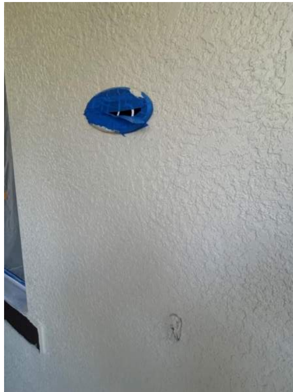
Figure 2: Installation of blue tape was completed around signs and details on the walls to protect from paint application.
