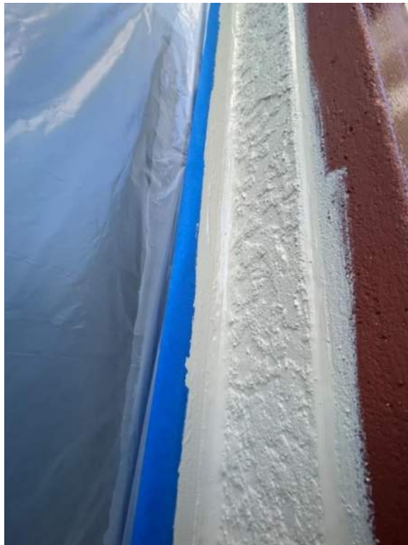
Figure 6: Stucco to metal sealant application was completed on the perimeter of all windows.
