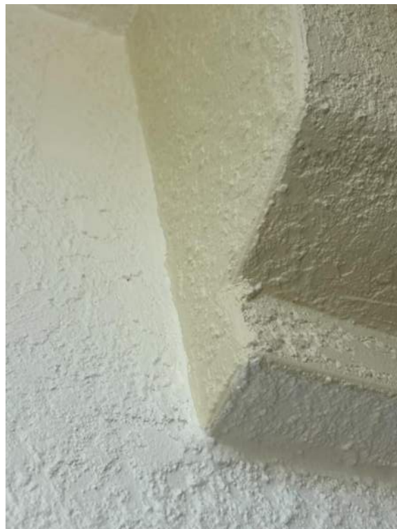
Figure 8: Stucco to stucco sealant application was completed around all corners and decorative bands.
