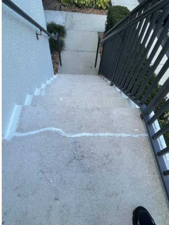
Figure 9: Crack repair was observed on the level 1 stair landings of both staircases in front of the building.
