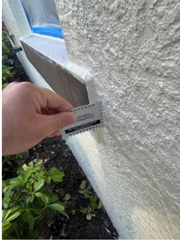
Figure 5: Wet film thickness test was completed for areas of ongoing paint application. Adequate mils was met according to specifications.
