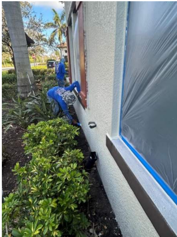
Figure 4: Cut-in paint application with brush was in progress on the west side exterior wall of the building.
