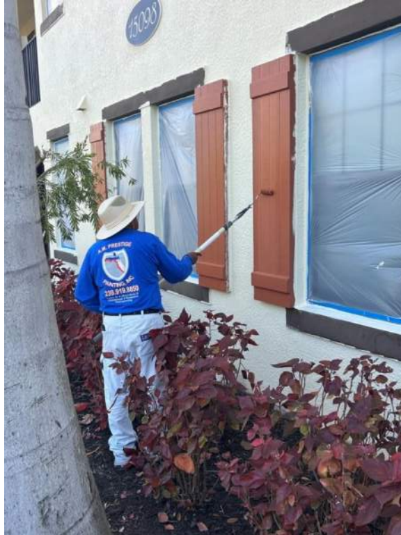
Figure 3: Roller paint application was in progress on the red details on each side of the windows.
