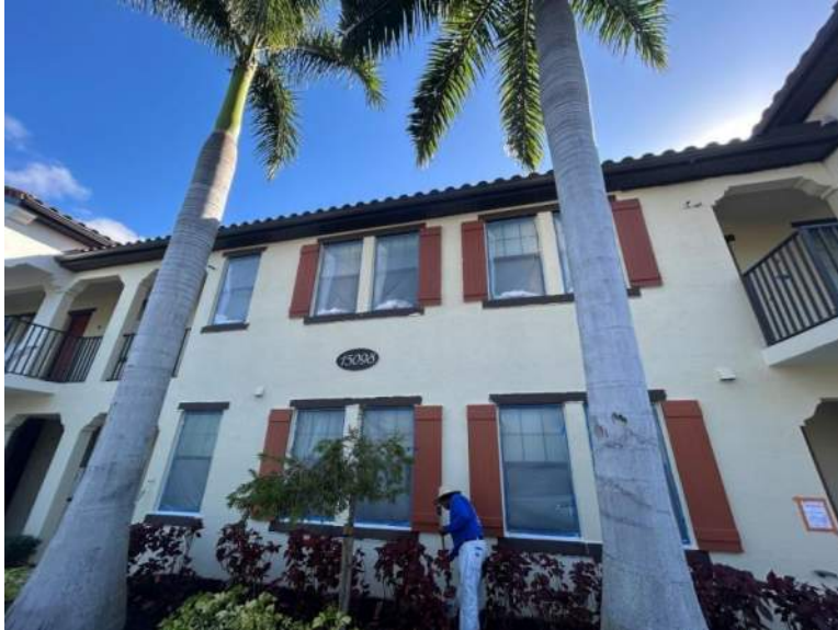
Figure 1: Installation of plastic was completed over all windows to protect from paint application.
