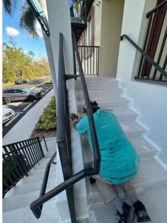
Figure 7: Stucco to stucco sealant application was in progress from the treads/risers to the wall of the south side staircase in front of the building.
