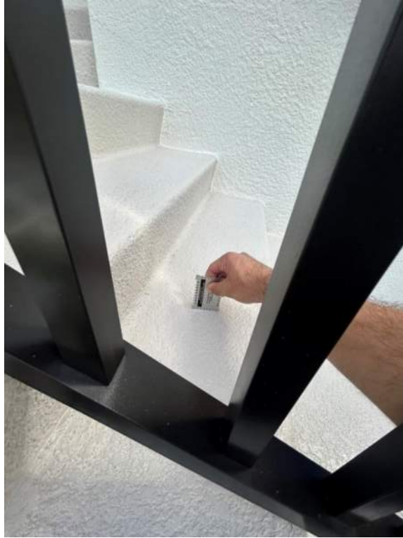
Figure 7: Wet film thickness test was completed for areas of ongoing paint application. Adequate mils was met according to the specifications.
