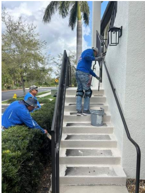
Figure 6: First coat of paint application was in progress on the left staircase.
