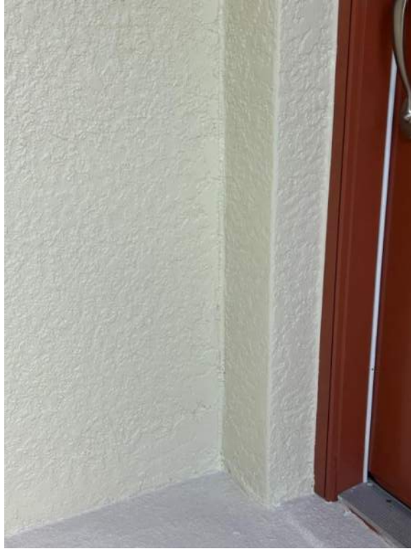
Figure 11: Stucco to stucco sealant application was completed on the vertical transitions of the building.
