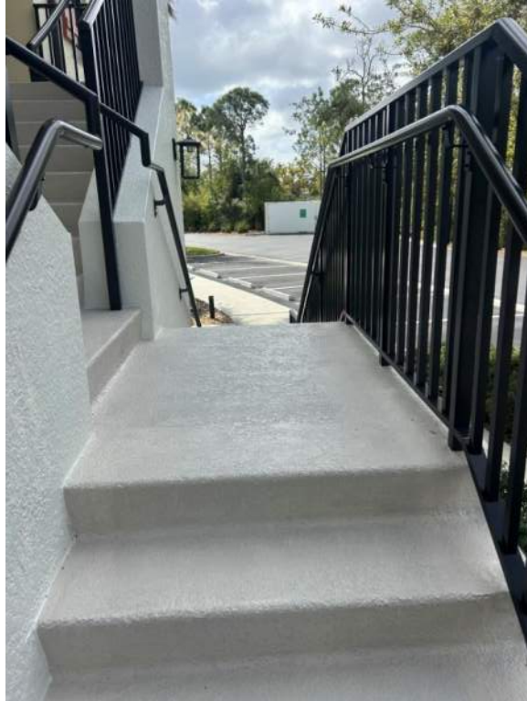
Figure 13: Crack repair was completed on the level 1 stair landings of both staircases in front of the building.
