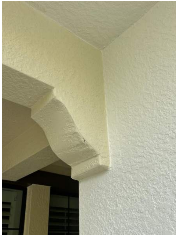
Figure 10: Stucco to stucco sealant application was completed around all corners and decorative bands.
