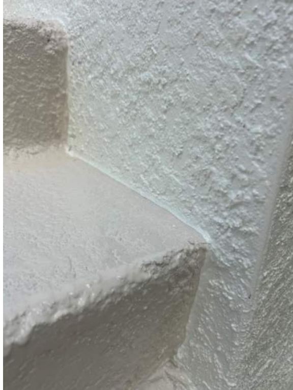
Figure 9: Stucco to stucco sealant application was completed from treads/risers to the wall of the staircases in front of the building.
