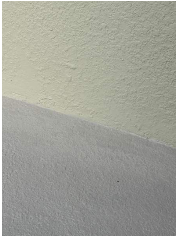
Figure 12: Stucco to stucco sealant application was completed from the walkway floor to wall.
