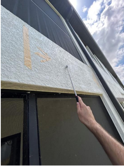
Right Side Stack 4
